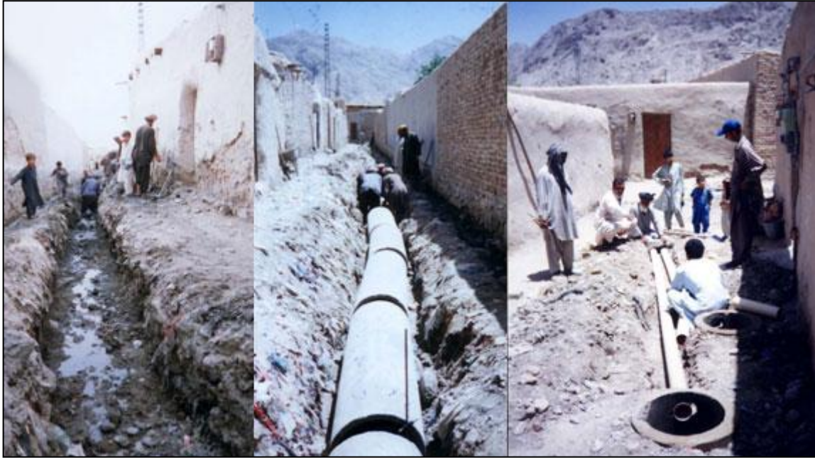
These pictures illustrate stages in the construction phase where all labour was part of the community contribution to the work. The pictures were taken in Qaiser Colony #1 (EFB area)
